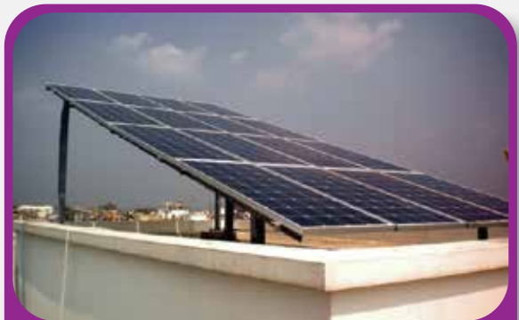
2.2KWp Solar On Grid System. Uttara, Dhaka.
