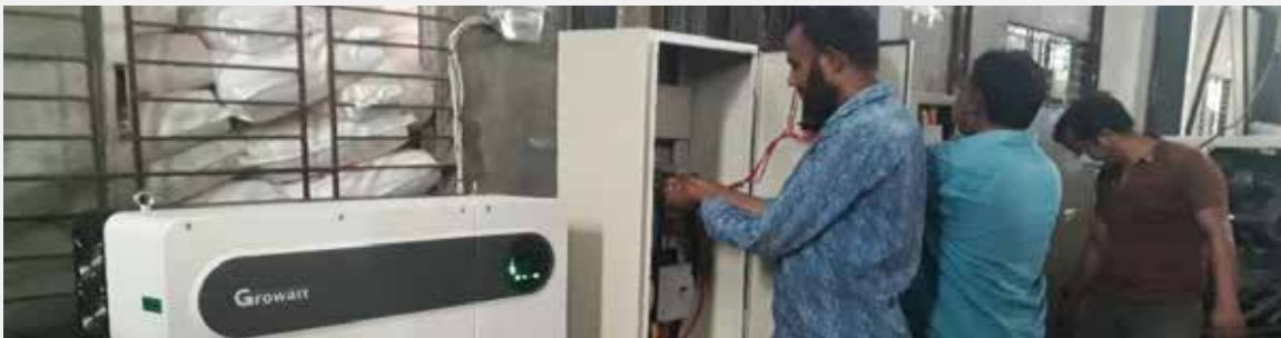
AC COMBINER BOX CONNECTION
