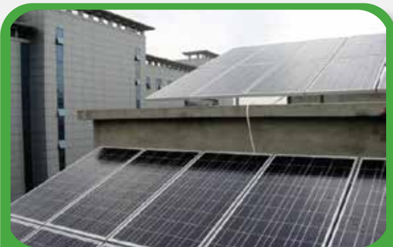
3.5KWp Solar On Grid System. Bashundhara R/A, Dhaka
