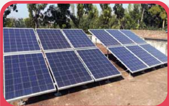
3KWp Solar On Grid System. Sitakunda, Chittagong.
