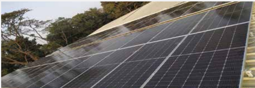
28.86kWp Solar Installed
