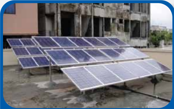
2.7KWp Solar On Grid System. Dhamandi, Dhaka.
