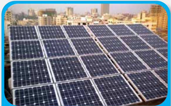
4KWp Solar On Grid System. Wari, Dhaka.
