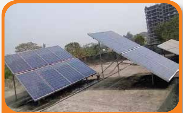
3KWp Solar On Grid System. Begumganj, Noakhali
